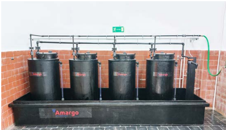
Laminated plastic tanks for laboratory liquid waste and low-level waste water
