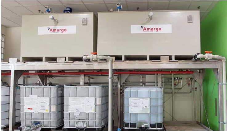
Intermediate tanks for Betaine and Aluminum Zirconium with installations
