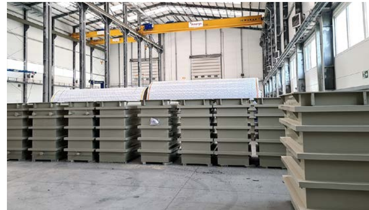
Process tanks (pickling tanks) with equipment and piping for automated production line of metal parts
