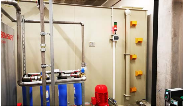
Fire tank for the archive building
