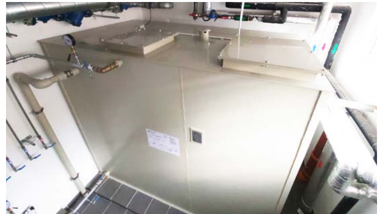
Drinking water storage tank for health center
